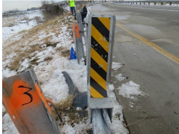
Figure 5. Guardrail end terminal impact, looking east
