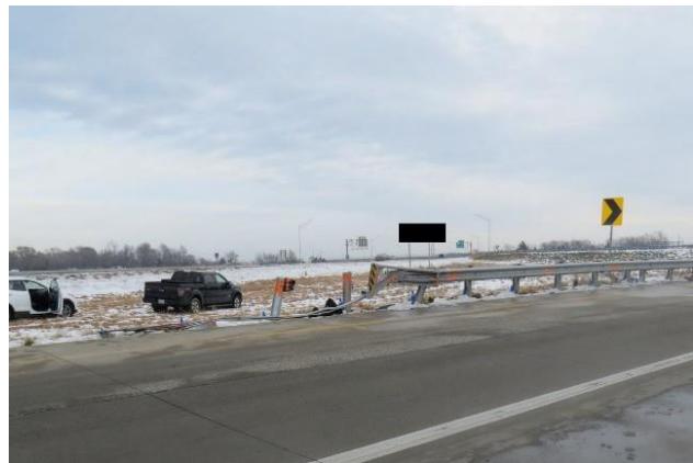
Figure 2. SoftStop guardrail end terminal, looking northeast
