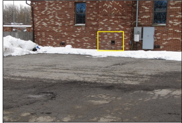
Figure 3. Southerly view of the area of the building struck by the Chevrolet
