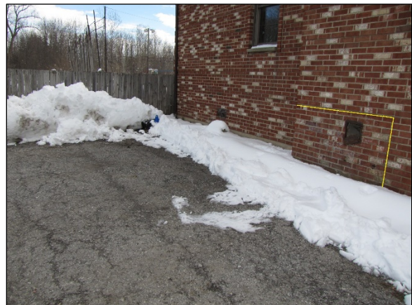
Figure 4: Southeast-facing image of the chimney impact and approximate final rest location of the Chevrolet
