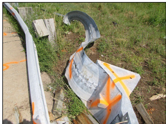
Figure 2. Guardrail ET2000 and extruded W-beam.
