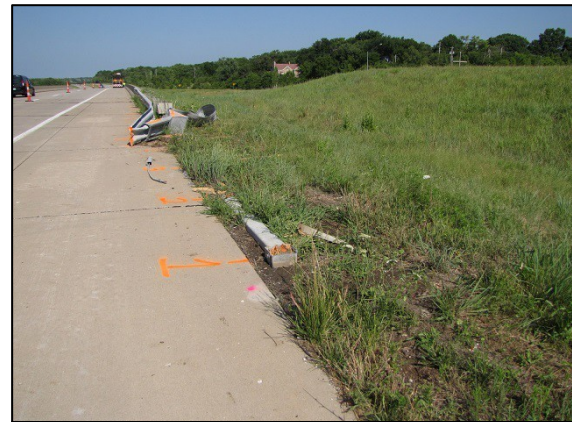
Figure 4. Area of impact, guardrail Post 1.
