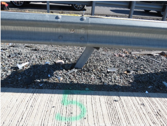
Figure 11. Easterly view of the bolt separation and displacement of Post 5
