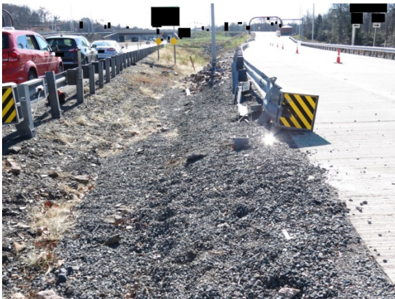
Figure 5. South-facing view of the struck SKT end terminal and guardrail system
