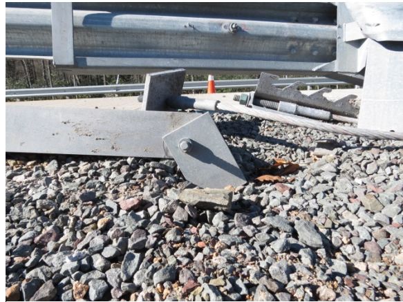
Figure 8. Westerly view of the displaced Post 2 at the hinge
