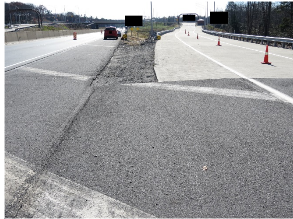
Figure 4. Southbound view of the Kia's approach to the guardrail impact
