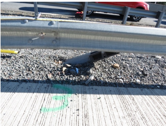
Figure 9. Easterly view of the displacement to Post 3
