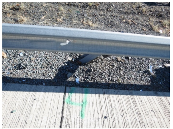
Figure 10. Easterly view of the bolt separation and displacement of Post 4
