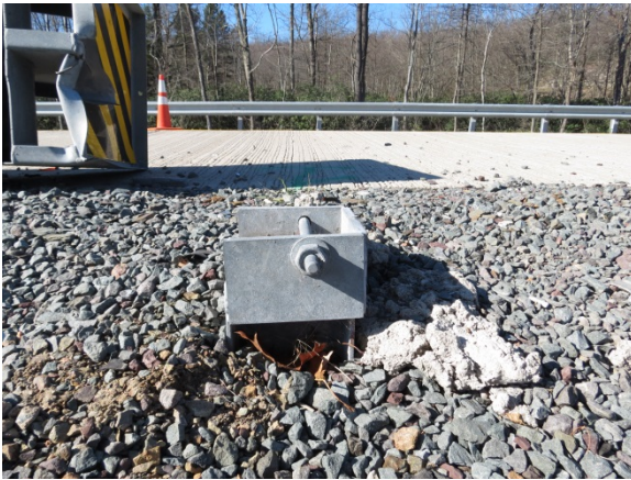
Figure 7. Westerly view of the displaced Post 1
