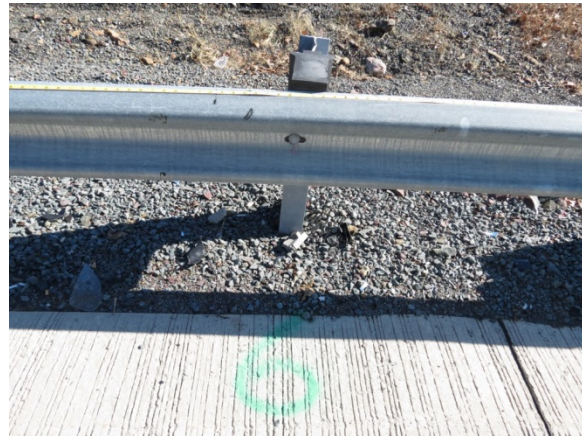
Figure 12. Easterly view of the minimal displacement of Post 6
