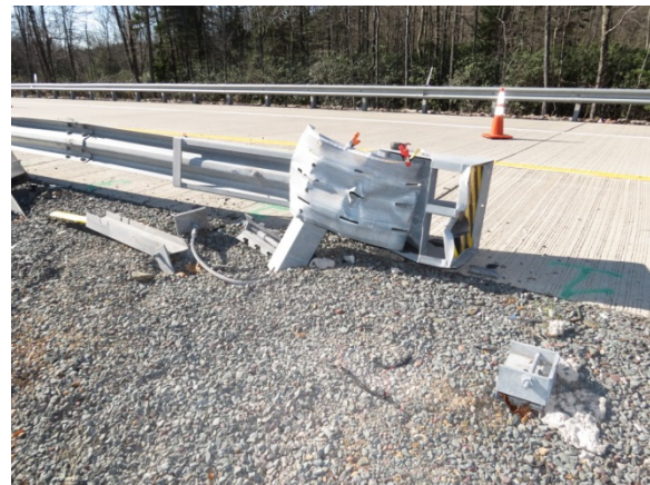
Figure 6. West-facing view of the extruded guardrail and displaced SKT end terminal
