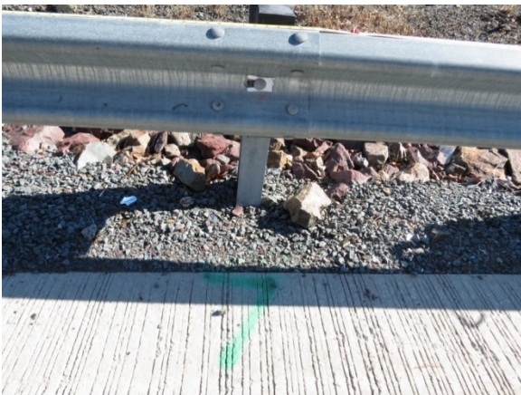
Figure 13. Easterly view of the system at Post 7
