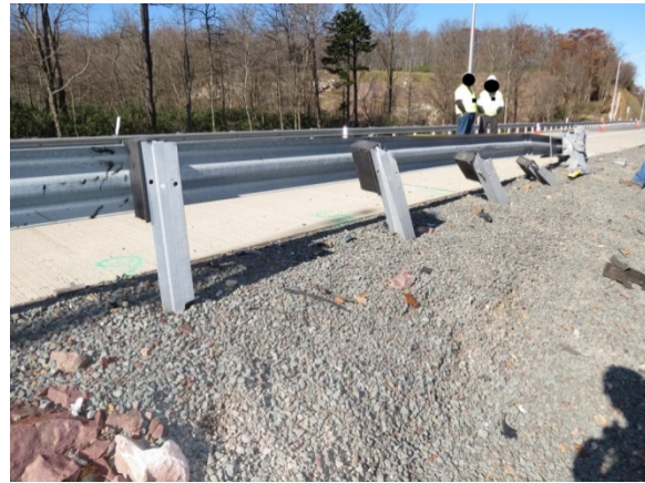
Figure 14. Northwesterly lookback view of the damaged guardrail system
