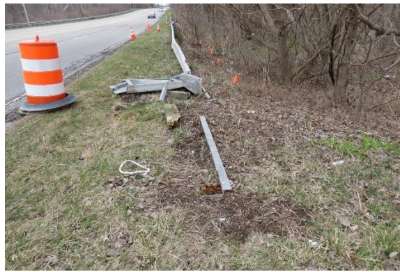
Figure 3. Area of impact with end terminal
