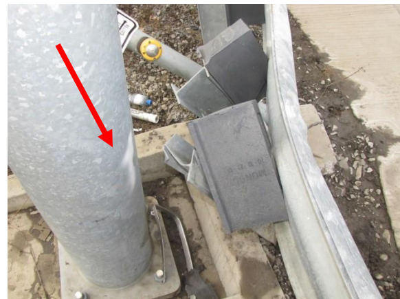
Figure 7. Close-up view of the deformed guardrail and the evidence of contact between the I-beam post and the pole (highlighted by the arrow)
