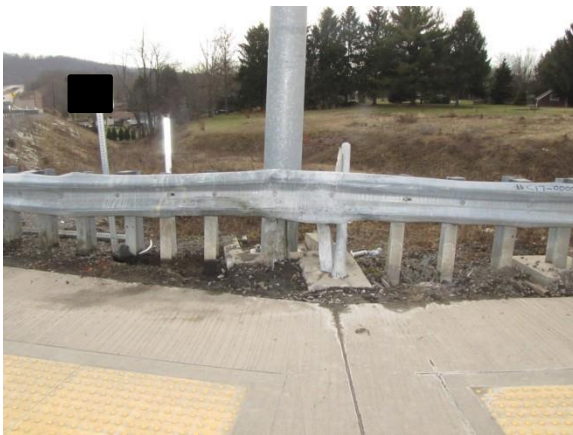
Figure 6. Southwest-facing trajectory view of the damaged guardrail
