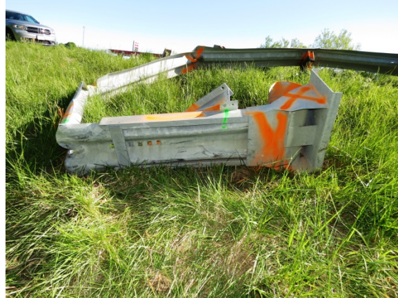
Figure 6. North-facing view of the impact head and deformed end terminal system lying in the area of protection at the time of the SCI crash site inspection
