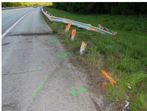
Figure 8. Southeast-looking view showing the damaged guardrail
