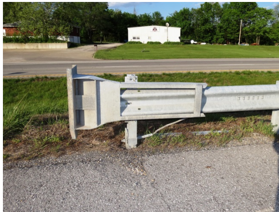
Figure 4. Image depicting an exemplar ET-Plus installation located on the opposite side of the roadway from the struck system
