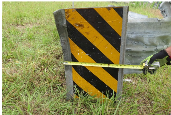
Figure 6. Direct damage to the face of the ET-plus
