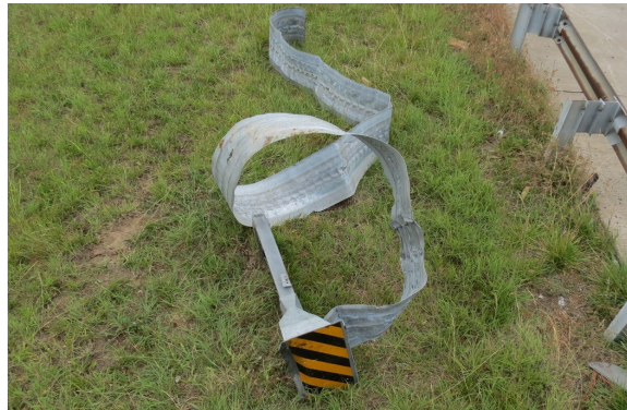
Figure 10. The damaged ET-Plus and extruded guardrail
