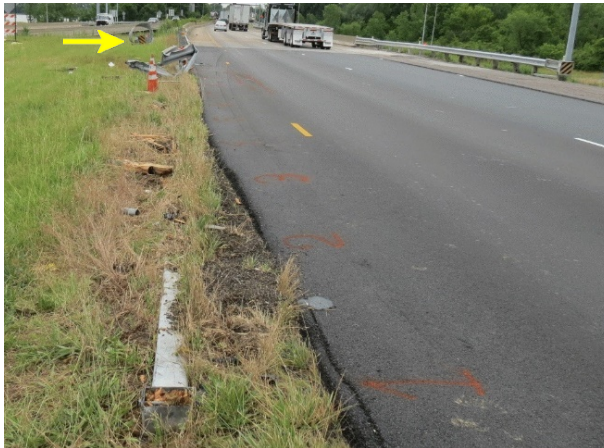
Figure 1. Overview of damaged guardrail and final rest position of ET-Plus (arrow), view east
