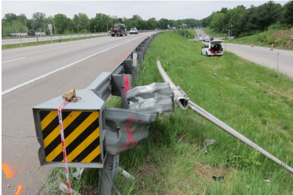
Figure 6. Southerly view of damage to the guardrail system and displaced luminaire
