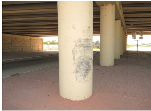
Figure 5. Point of column impact (Event 3) looking south
