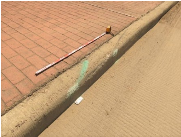
Figure 4. Point of curb impact (Event 1) looking south
