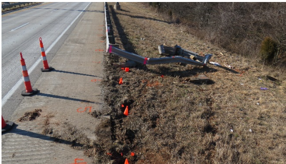
Figure 1. The damaged guardrail and guardrail head, view west
