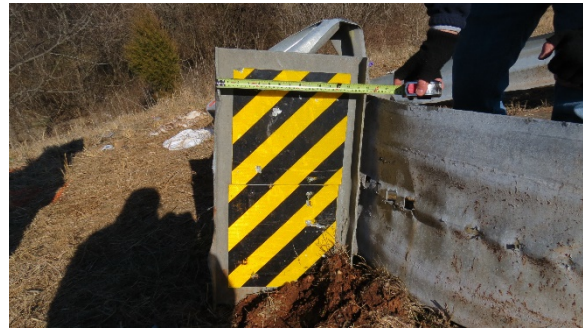
Figure 7. The face of the guardrail head struck by the Pontiac
