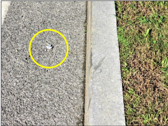
Figure 4. Impact to the curb from the Jeep's front axle (Event 3) and metallic fragment
