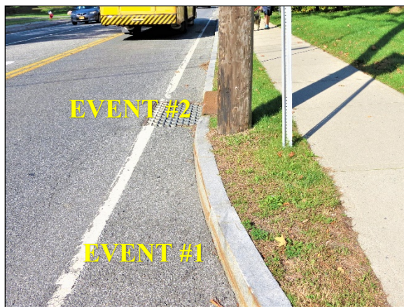
Figure 3. North-facing view of the impacts to the curb and utility pole
