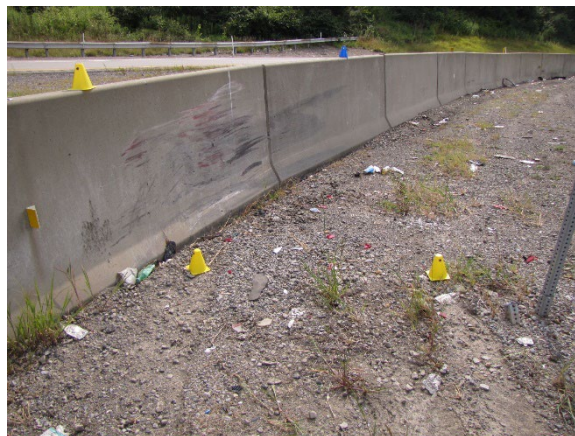
Figure 5. Southwest-facing image of the barrier showing its impact damage
