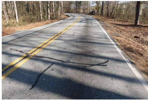
Figure 2. Northbound view of the crash site.
