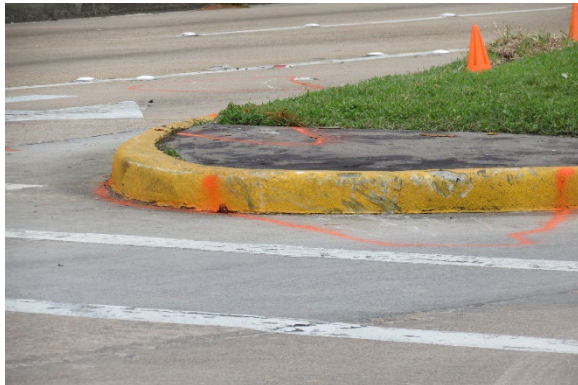
Figure 4. West median tip, struck by right rear top of the ambulance
