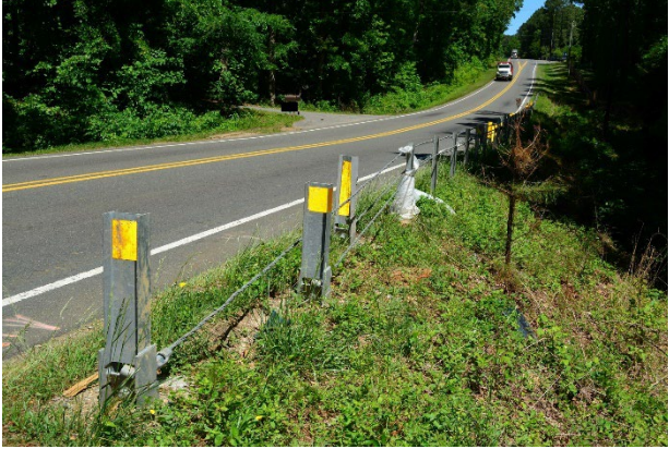
Figure 5. Facing north and the forward section of the first CBS, the second post from the left is the first object struck for Event 1
